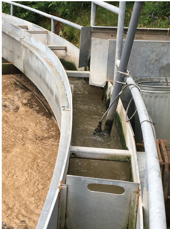
FAR LEFT: Bryce Stewart, engineer in training with Island Water Technologies, installs an in-line Sentry sensor in the influent channel using a PVC rail mount. NEAR LEFT: The Sentry sensor in the influent channel is attached to PVC pipe with U-bolts and fixed to a rail. The sensor connects to an online dashboard, enabling operators to monitor remotely for shock loads and other events affecting the plant.
